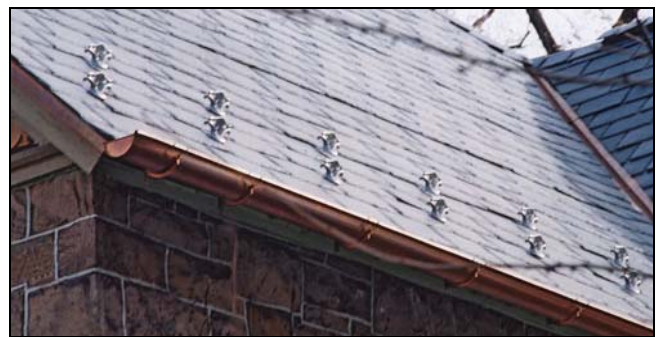
Snow birds provide protection and a visual pattern at the edge of this roof. Note the half-round gutter installation.
