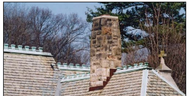
The steeply pitched slate roof, large chimney and the ridge cresting add visual interest to this building.
