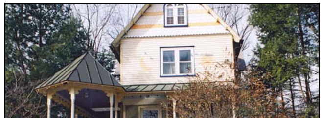
Standing seam metal roofing can be found at steeply pitched roofs, while flat seam metal roofing is more typical at shallower roofs.
