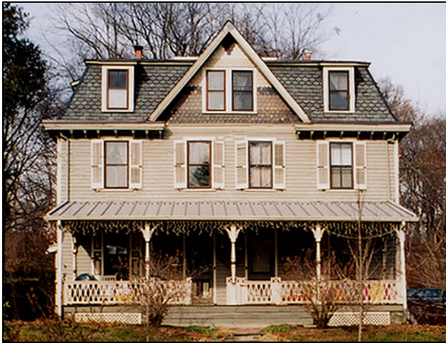
The slates on this Mansard roof were replaced with dimensional asphalt shingles to replicate the color and pattern of the original.
