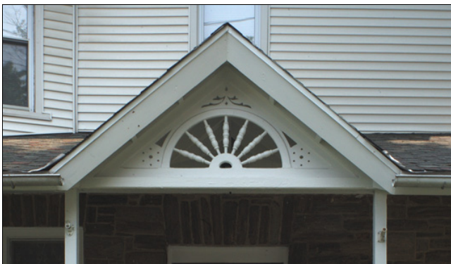
Although the walls of this residence were covered with artificial siding, the decorative wood pediment remains exposed to view.
