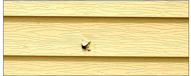
If considering artificial siding, a smooth finish is recommended rather than a wood-grain finish. Replacement of this aluminum siding section would be the best way to repair the puncture. Since siding colors tend to fade from sunlight, the replacement siding probably will not match the existing siding.
