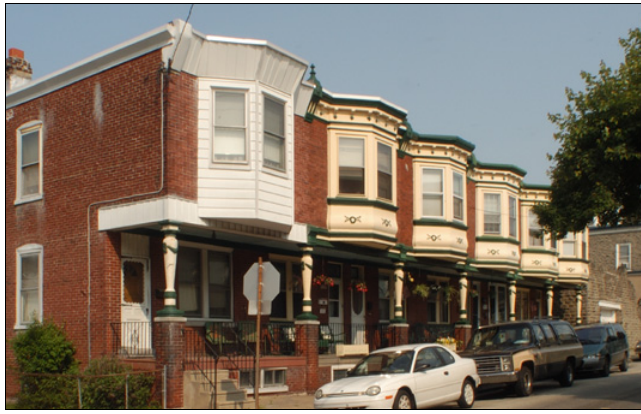
Artificial siding over decorative elements can greatly change the appearance of the streetscape. The artificial siding can trap moisture and deteriorate the underlying woodwork.
