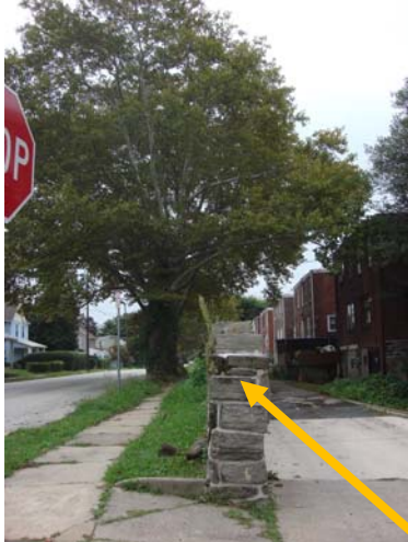
Wall shifting in many areas creating potential unsafe situation
