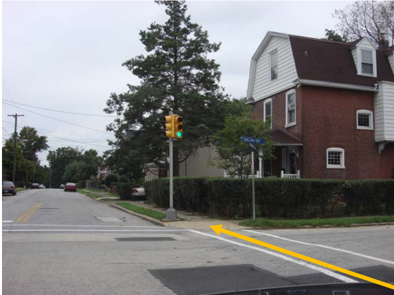
ADA ramp not up to code
