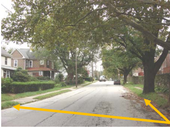
Low and failed curbing
