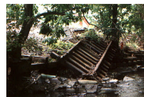
7. SEPTA leave its debris behind after track repairs. Action/BMP : Township will work with SEPTA to clean it up.
