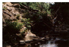
6. Dumping along the Creek bank destroys the potential for a riparian buffer to flourish, and it is unattractive. Action/BMP : Determine who is routinely dumping.
