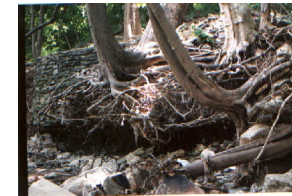
4. Tree roots are exposed along the steep banks behind the Wyncote Post Office due to severe runoff from surrounding parking lots of the train station and post office. Action/BMP : Consider an infiltration system at the end of the Jenkintown train station parking lot and post office.
