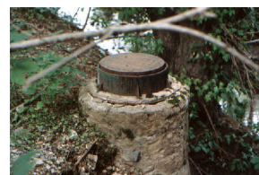
8. Exposed manhole from Tookany Creek bed down cutting and erosion. Action/BMP : Develop a program to inspect, repair and maintain manholes that are exposed.
