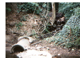
9. Dumped construction material along the banks, and invasive ivy prevent the riparian buffer from flourishing. Action/BMP : Determine who is routinely dumping to clean up, and replant the riparian buffer.
